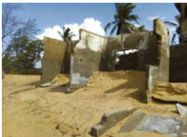
Wall sections of houses ravaged by the sea
