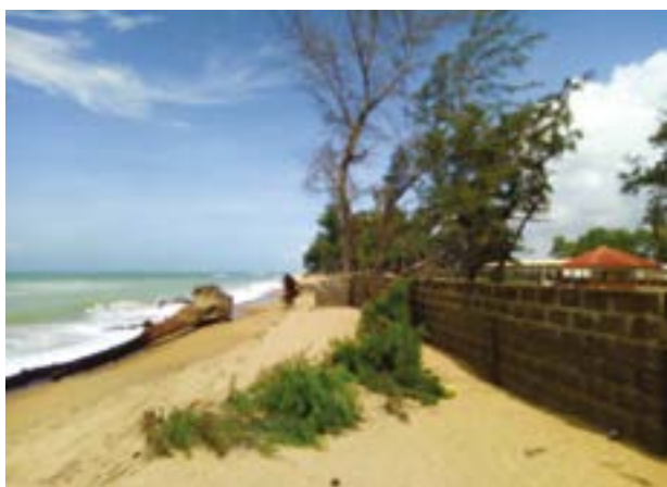
One of the four sides of the walls of one of the houses ravaged by the sea
